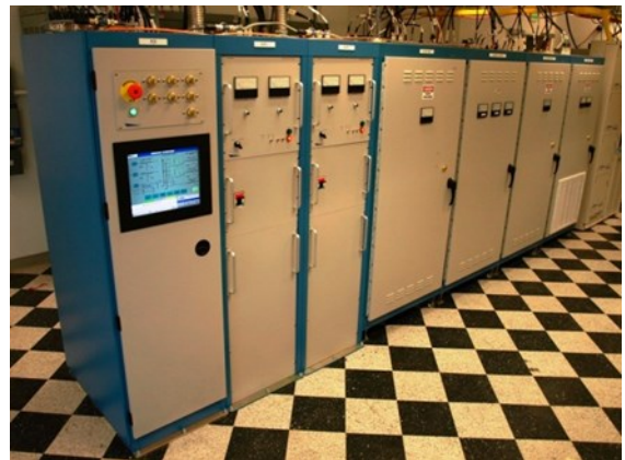
Figure 1. Installed Shore Power Feed Equipment.
