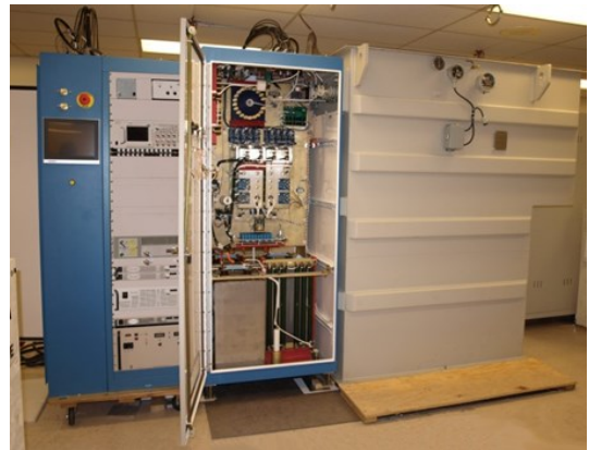
Figure 1. DTI's prototype solid-state ESS-class klystron modulator, developed under a DOE SBIR grant. This design is optimized for long pulse operation with highest possible reliability and availability required for particle accelerator user facilities and test stands.
