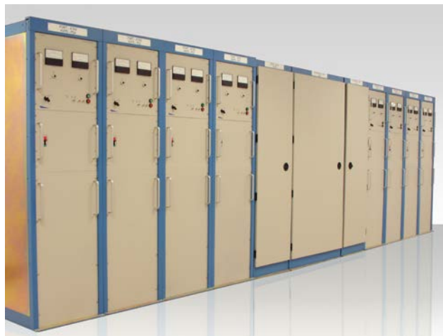
Eight 200 kW shipboard DTI PowerMod™ Power Supplies and 480 VAC power distribution as installed for the Cobra Judy S-Band Phased Array Modernization.
