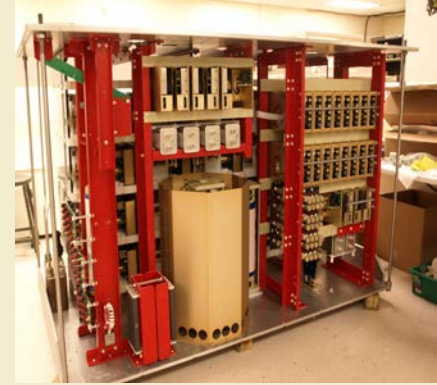
DTI Marx Modulator. Twenty 6 kV "core" switch modules erect a 120 kV output pulse when placed in series. Sixteen 900 V "corrector" switch modules address droop over the 1.5 ms pulsewidth.
