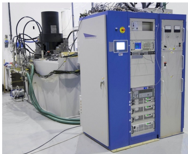
Fig. 1. Installed Daresbury modulator, consisting of a controls rack, electronics rack, high voltage power supply and modulator tank
